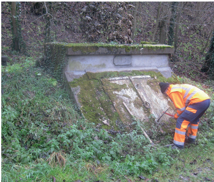
Abb. 32: Mittlerer Quellschacht mit Behälter in Amoltern. Foto: B.G., 20.12.2016. Fig. 32: The middle spring chamber with reservoir located in Amoltern.
