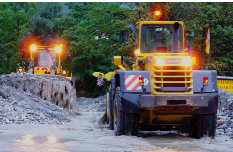
Fig. 3: Deployment of heavy machinery to clean up sediments and rubbish after debris flows. Source: municipality of Pfunds.
