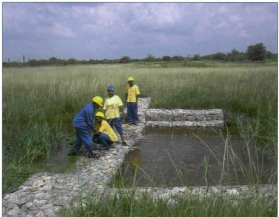
Fig. 10: Working for Wetlands staff evaluating the completed gabion structure and its positive effect on the eroded gully in the Molopo peatland. Picture by Piet-Louis GRUNDLING.
